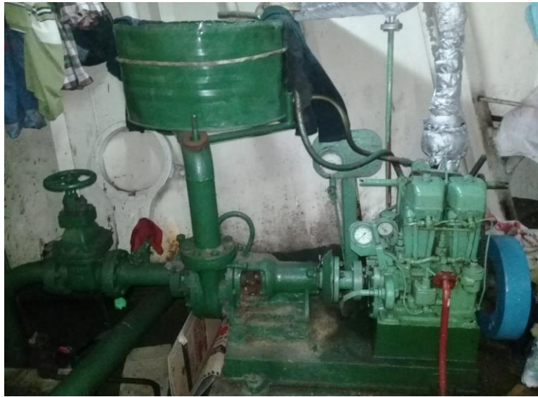
Gambar 4.2 Emergency fire pump
