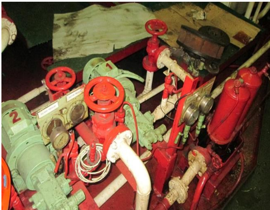
Gambar 1. Circulation Pump Unit
