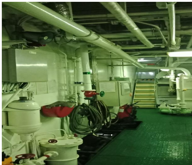
Gambar 5 Selang Hydrant ( Documen Kapal BC 60001)
