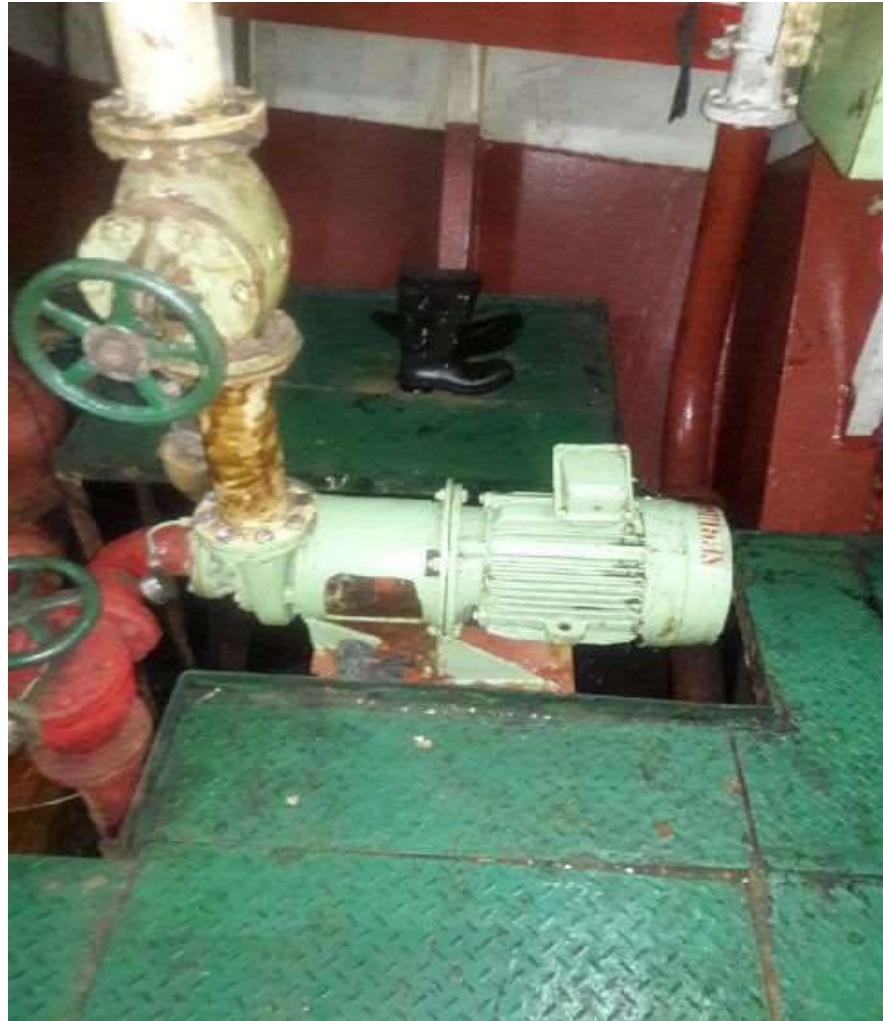
Gambar 2.4 Sea Water Scrubber Pump
