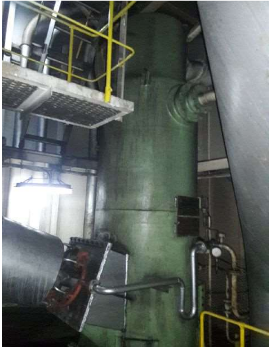
Gambar 2.3 Inert Gas Scrubber
