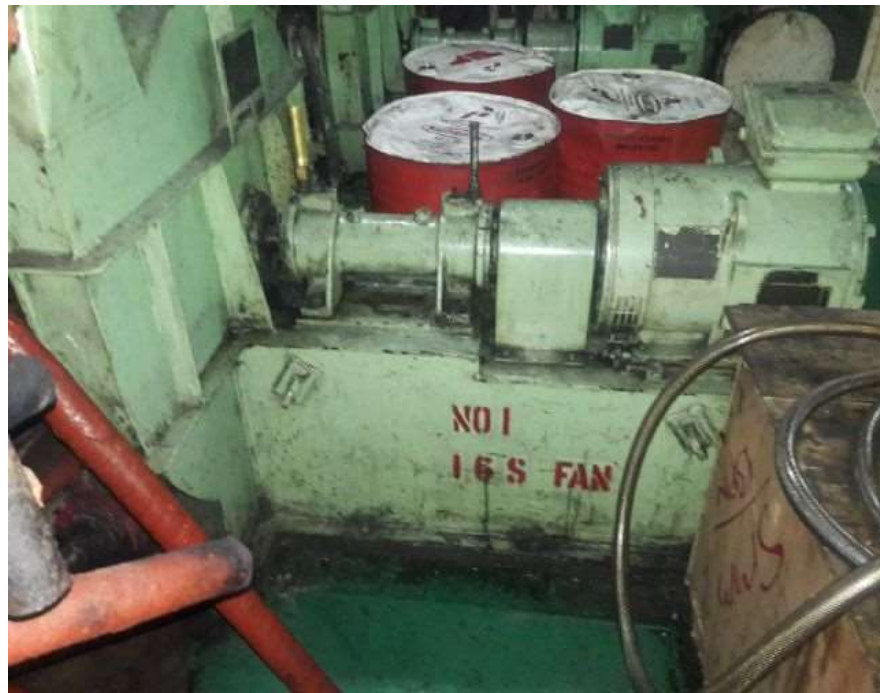
Gambar 2.5 Inert Gas Blower Tampak Samping
