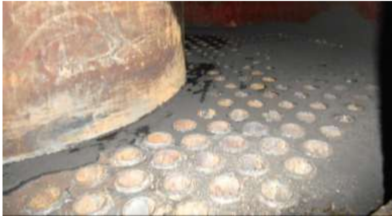
Gambar 2.5. Pipa Boiler (MV. Sinar Papua)
