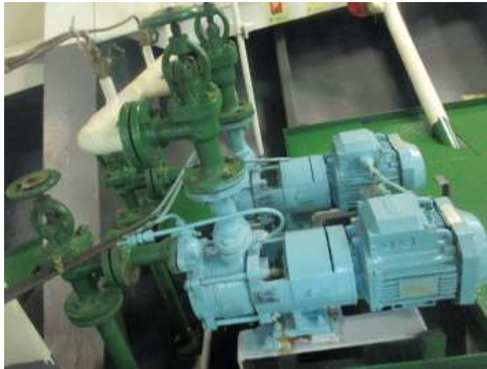
Gambar 7. Deck Water Seal Pump
