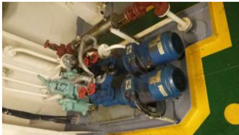
Gambar 4. Fuel Oil Pump
