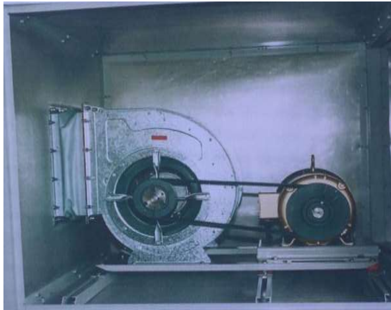
Gambar 6. Blower AC (Sumber: KM. SIMORE)
