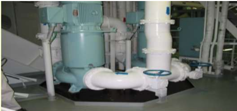
Gambar 2.3. Jacket Cooling Fresh water Pump
