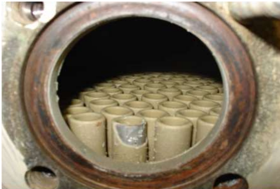
Gambar 7 Evaporator Heat Exchanger
