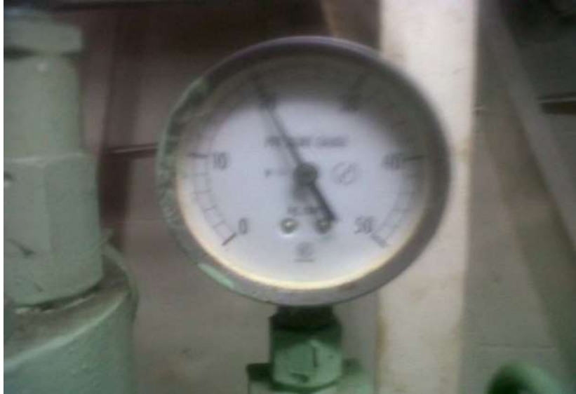
Gambar 2.3 Manometer. (KM, Indah Virgo)
