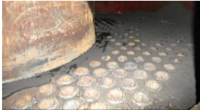
Gambar 2.5.Pipa Boiler (MV. Sinar Papua)
