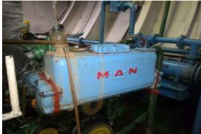
Gambar 2.5 Fresh water cooler tank
