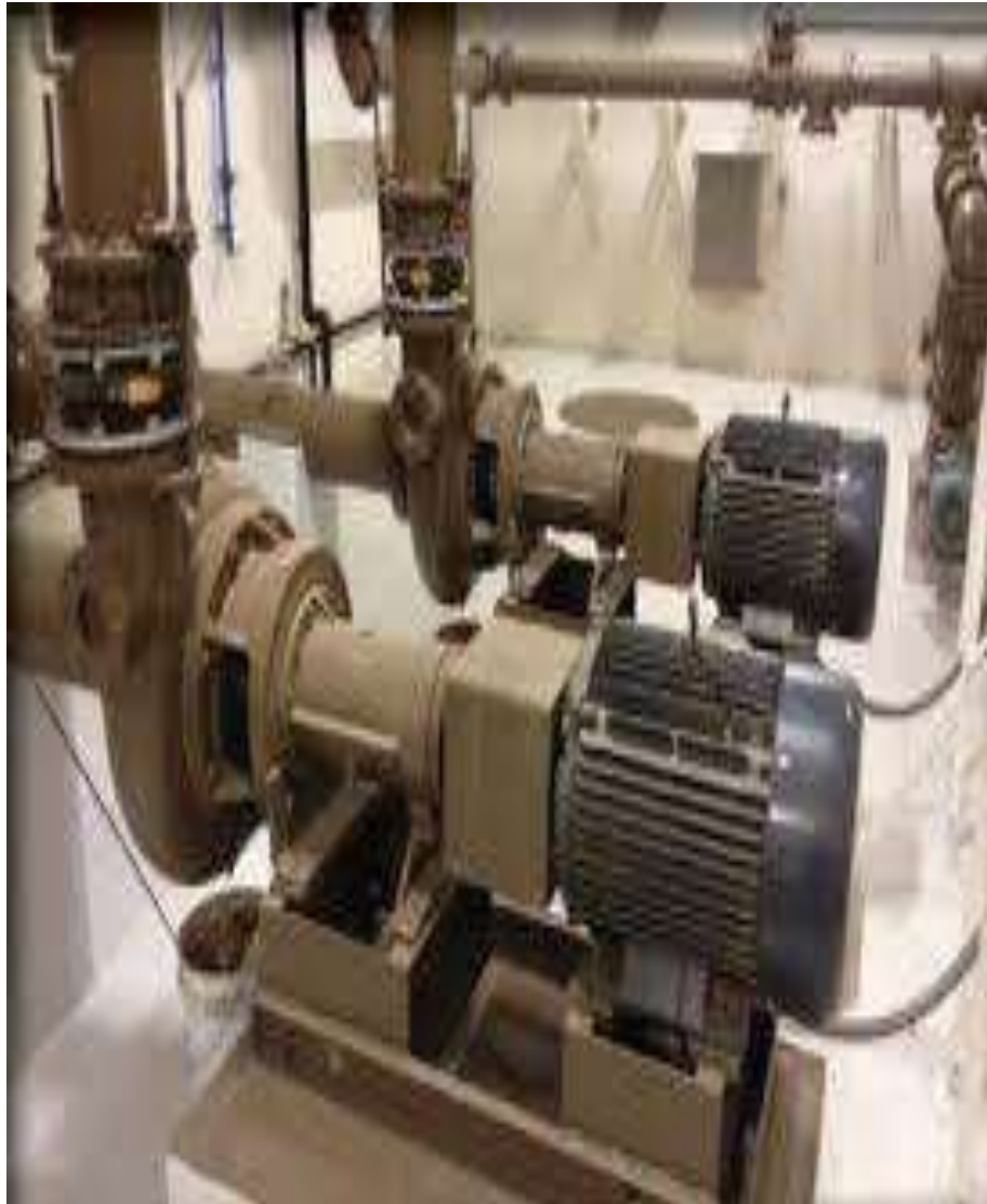
Gambar 2.4 Sea Water Scrubber Pump
