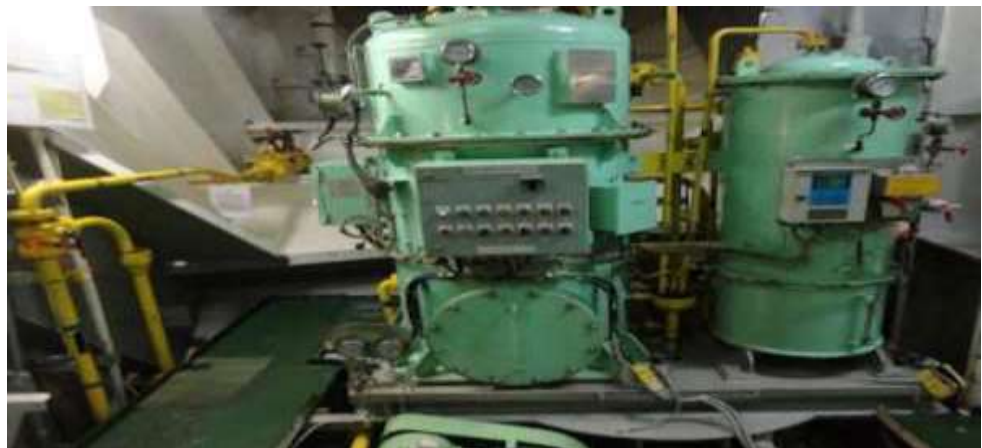
Gambar 1 oil water separator
