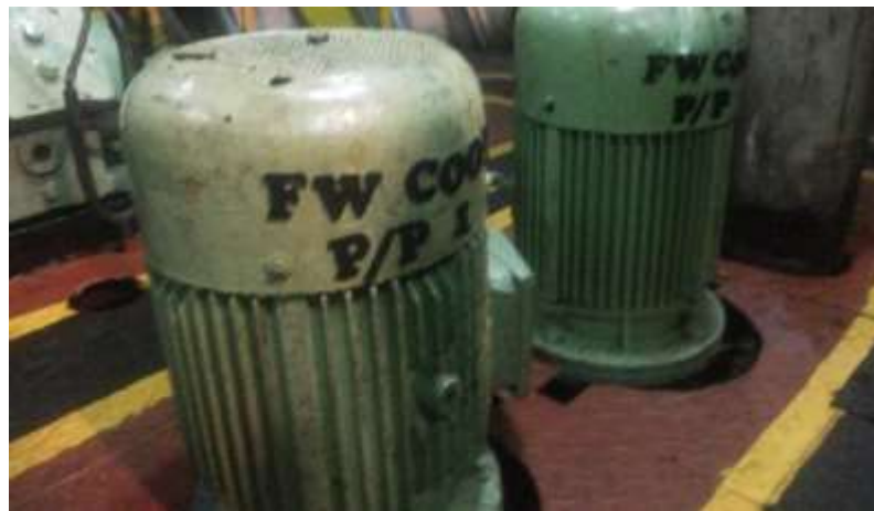
Gambar 6 Pompa Fresh Water KM.Sinar Papua
