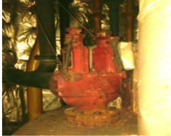
Gambar 2.8. Safety Valve Sumber : MV. INTAN DAYA 368
