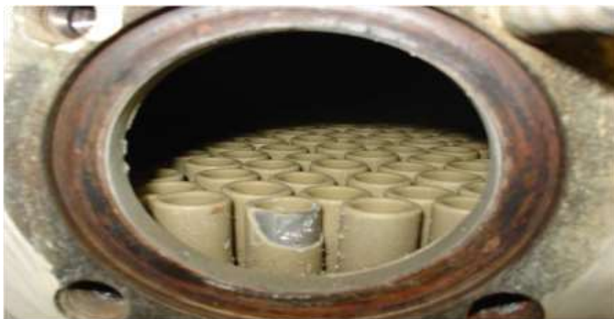
Gambar 4 Evaporator Heat Exchanger
