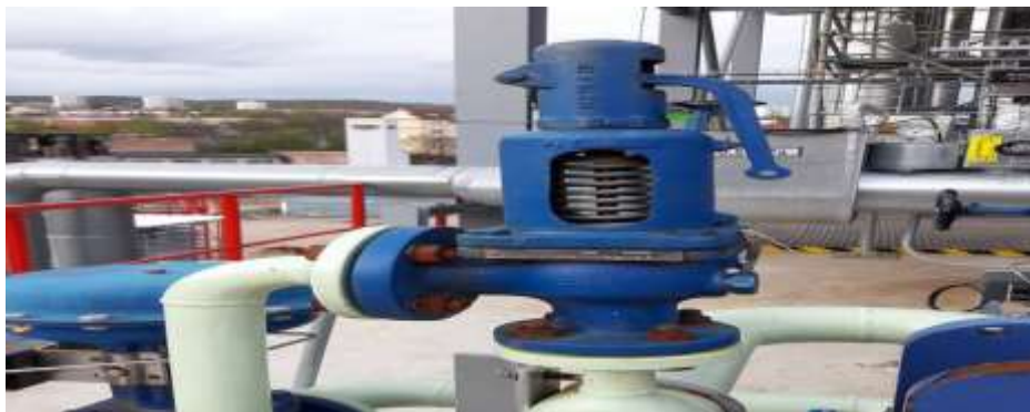
Gambar 7. Safety valve economizer
