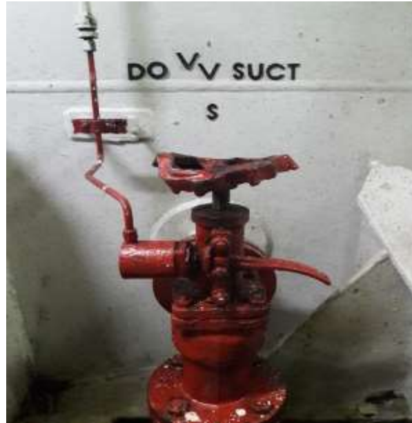
Gambar 2.6 M.D.O storage tank quick closing valve (starboard side) ( Sumber: Dokumentasi penulis )
