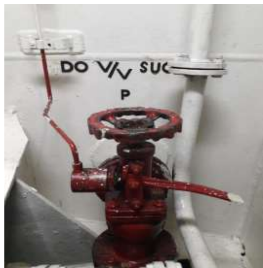
Gambar 2.7 M.D.O storage tank quick closing valve (portside) ( Sumber: Dokumentasi penulis )
