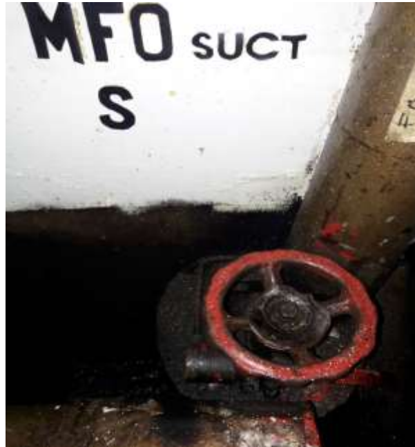
Gambar 2.2 M.F.O Storage tank quick closing valve (starboard side) ( Sumber: Dokumentasi penulis )
