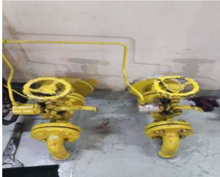
Gambar 2.10 L.O storage tank quick closing valve ( Sumber: Dokumentasi penulis )
