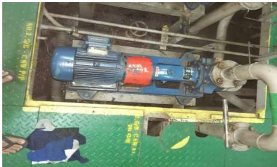
Gambar 2. Pompa Fresh Water
